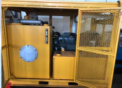
Hydraulic Power Pack
